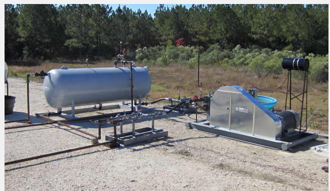
Tally's permanent installation after production testing with a natural gas unit.
